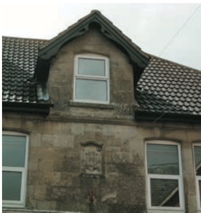
An example of a Victorian dormer formed in dressed stone with a decorative and preformed timber bargeboard.
