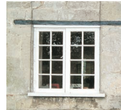
Casement window with timber lintel. Length of lintel suggests windows have been modified at some stage.
