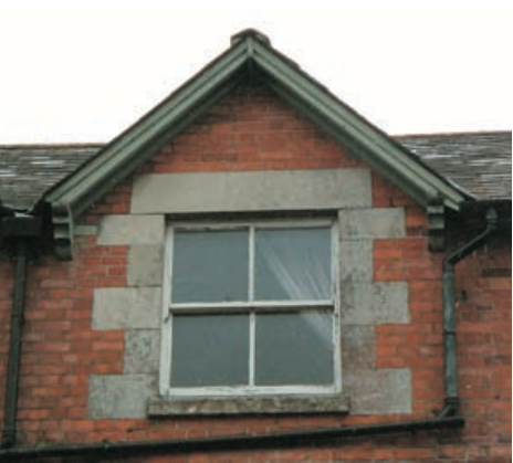
Victorian gable detail opening formed with stone window detail. A simple decorative timber bargeboard on brackets.
